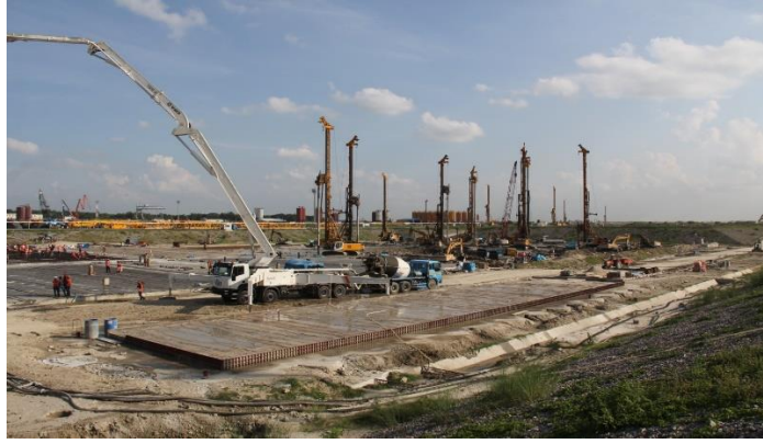
Figure 3: Completion of Reinforcement works ready for First Concrete Pouring Unit-2 of Rooppur NPP
