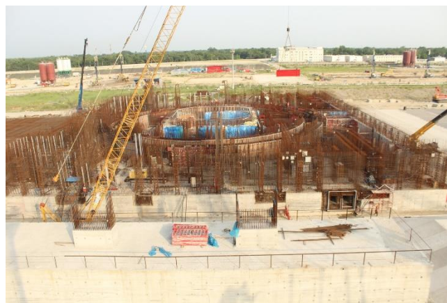
Figure 2: Construction activities at the Unit-1 of Rooppur NPP up to the ceiling level of 0.000
